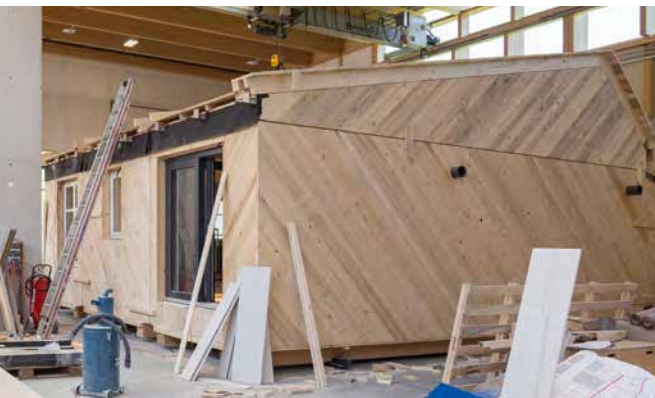
Diagonal formwork made of solid wooden boards by the team from Karlsruhe. © RoofKIT / SDE 21/22
