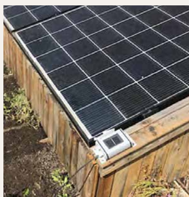
Irradiation measurement at module level with calibrated solar cells. Buildings with PV systems facing different directions were equipped with multiple sensors © SDE 21/22
