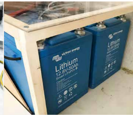
2.5 kWh battery storage by the team from Eindhoven © SDE 21/22
