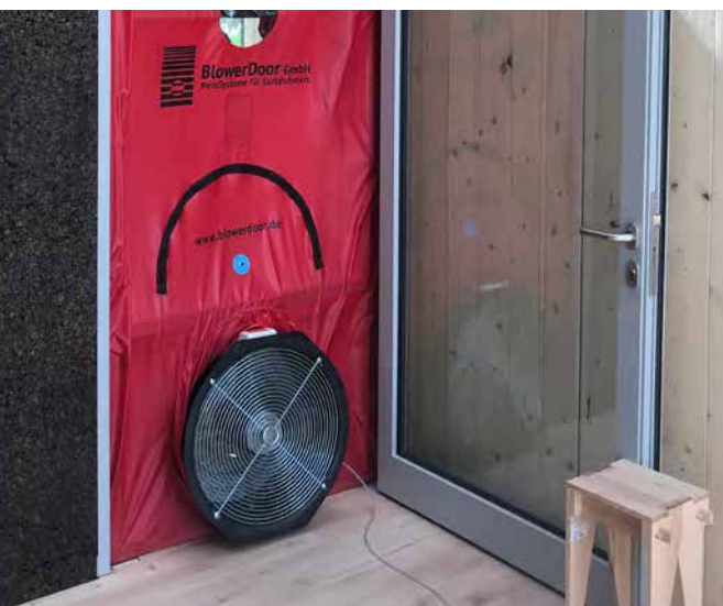
The airtightness of the building envelope was checked for each house using a "blower door". © SDE 21/22
