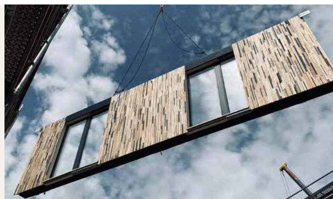
Façade element with preinstalled cladding and windows by the Team from Stuttgart. © coLLab / SDE 21/22
