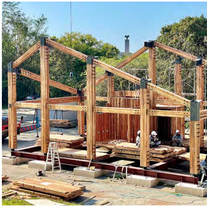
Timber frame made of cedar as the primary load-bearing structure. The Taipei team used small-scale elements.
