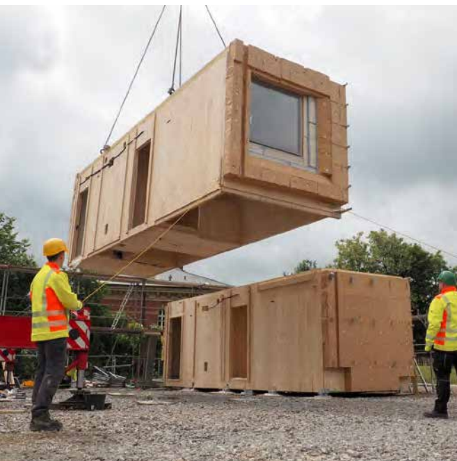
Module assembly by the team from Aachen: The second of six room modules in total is assembled. © LOCAL+ / SDE 21/22
