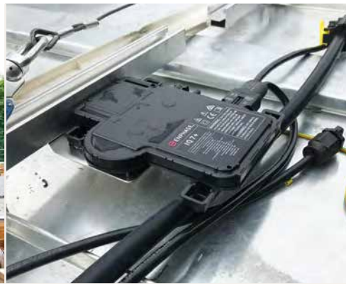
Module inverters with 290 W p by the team from Grenoble © SDE 21/22
