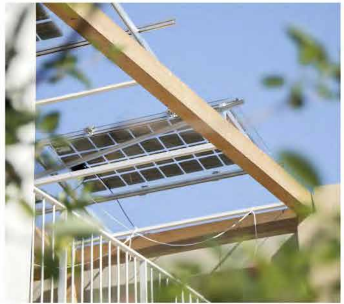
Solar panels detail
