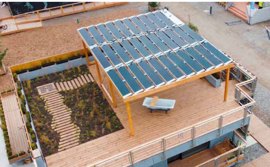
Thin-layer photovoltaic films on the roof pergola - photo from south-east
